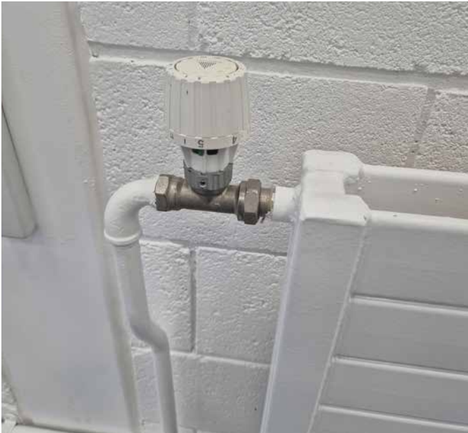
Original inefficient valves
